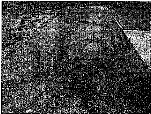
Photo 35 - A portion of the court has tree root damage that may be a hazard
