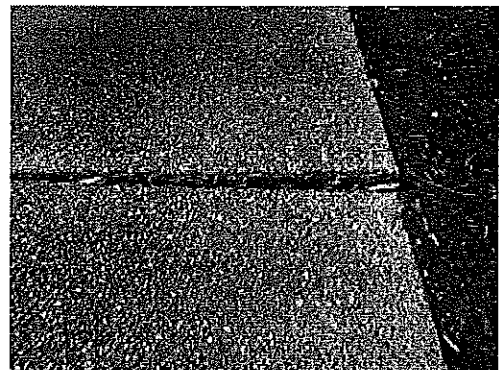
Photo 4 - There is one significant trip hazard near the pool walk
