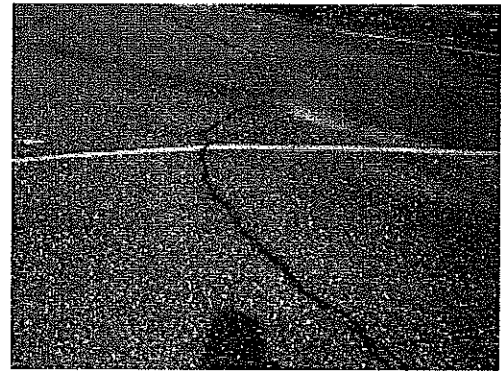
Photo 36 - The asphalt court has several large cracks
