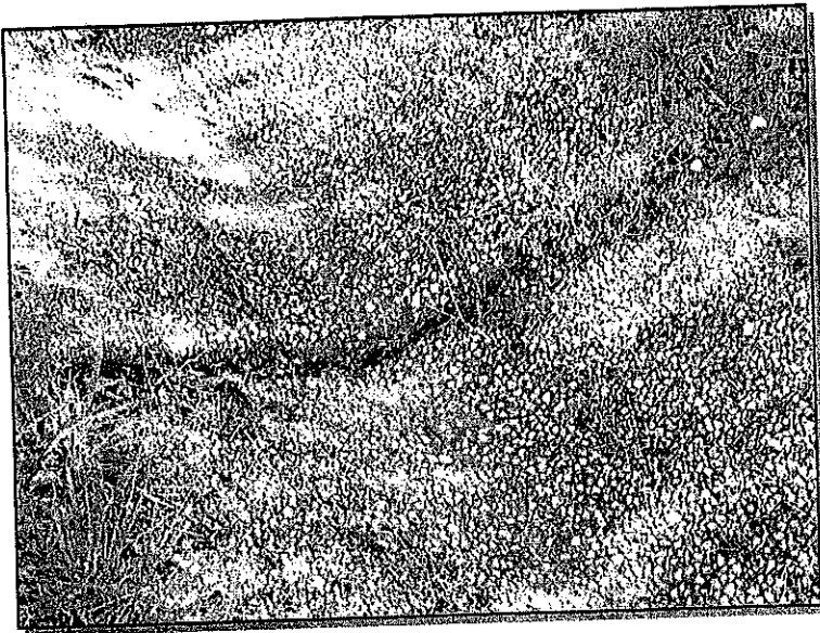
Concrete drainage swale settlement
